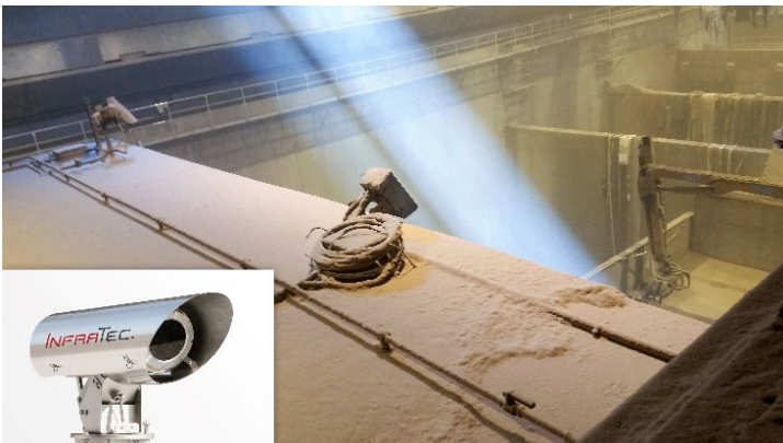
Fig. 1: Permanently installed infrared cameras are used for monitoring the hopper.
