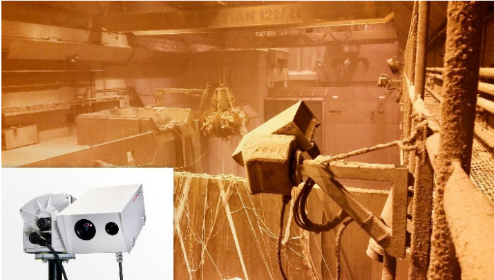
Fig. 2: The combination of pan/tilt heads, infrared cameras and visual cameras offers an excellent overview of the material located in the various stacking compartments.
